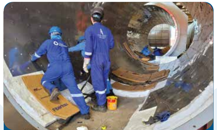
WHRU Exhaust Insulation
